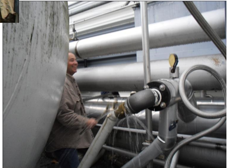
Recovery Compressor temporary cooling water hoses
